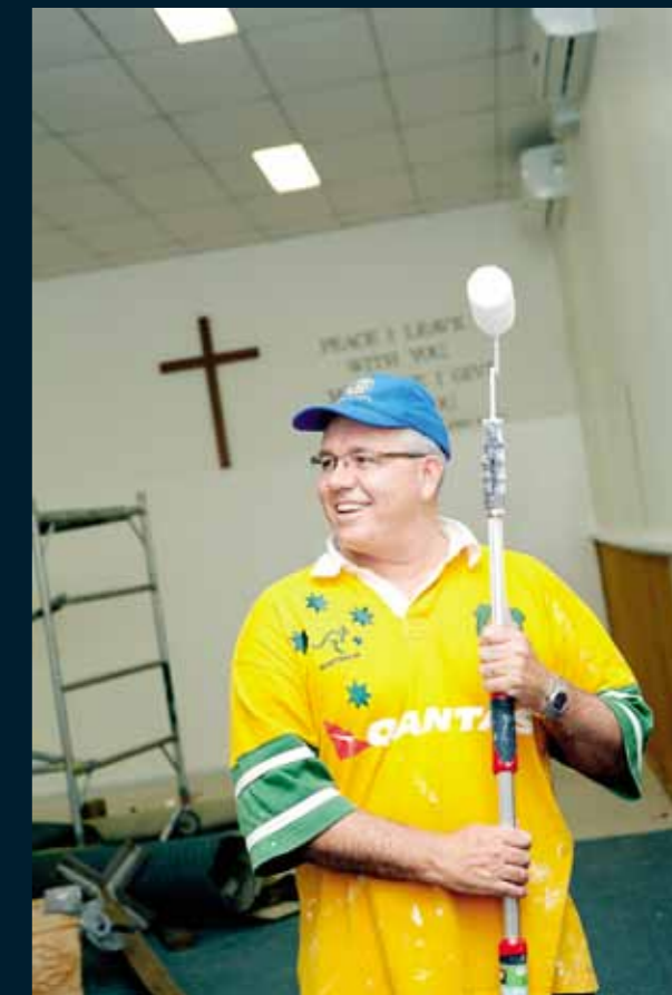
Envoy Penny Williams (left) serves at the Cafe De Light that operates out of the Armidale Corps complex, which has recently undergone major renovations. Lieutenant Ged Oldfield (above) puts the finishing touches on the citadel walls.
